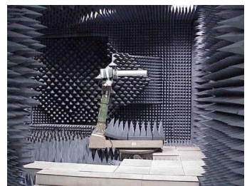
Antenna Patterning Chamber
